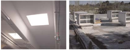
Figure 2. (Left) Inner view of the light pipes located between the beams. (Right) Outer view of them.
