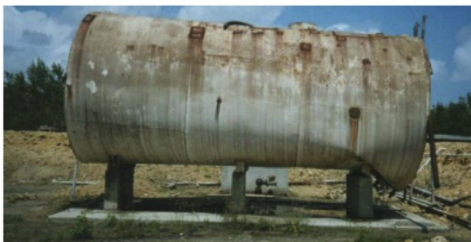
Fig. 1. Buckled tank with three saddle supports, Peñuelas, Puerto Rico (Photograph by LAG).
