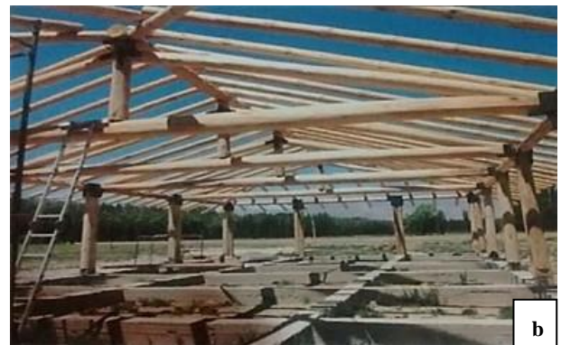
Figure 8: Multi-Purpose Centre construction details. a- excavating the foundations b- tie-beams and elevation of interior floor.
