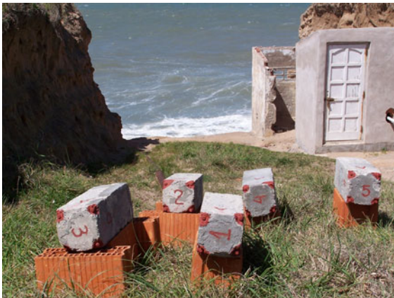
Fig. 1 Exposed reinforced concrete members
