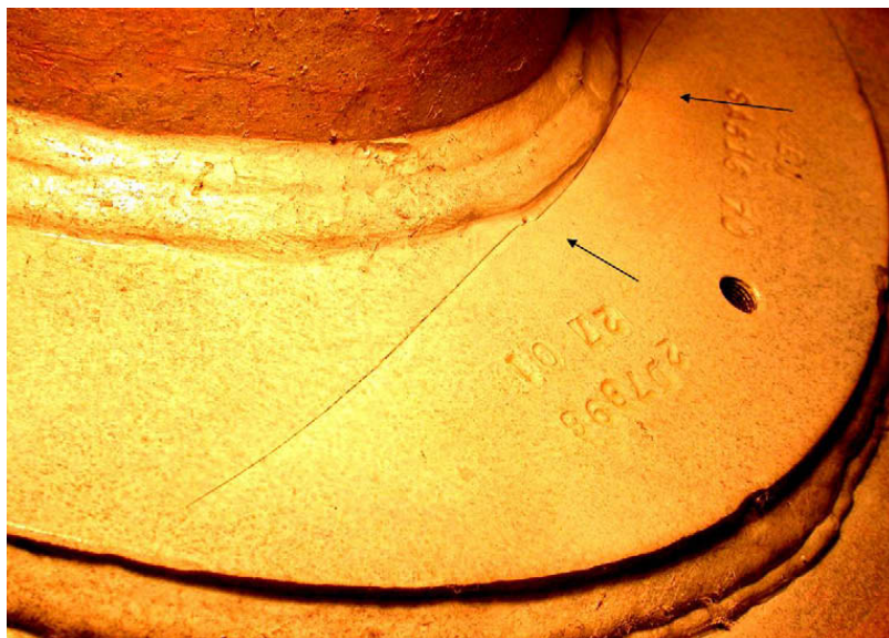
Fig. 11. Case 3: Crack initiation in the reinforcement saddle of the flange in suction vessel.
