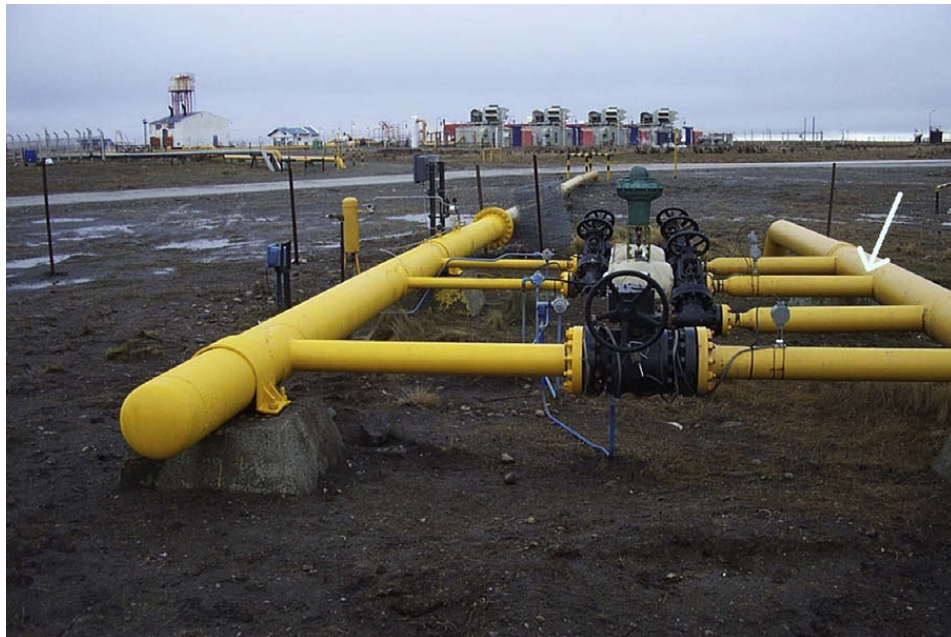
Fig. 5. Case 2: Location of element failed in collector pipe.
