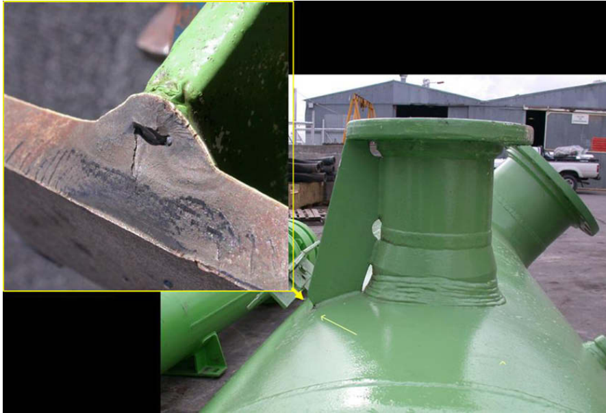
Fig. 3. Welded flange in the second vessel, replacement of the failed vessel.
