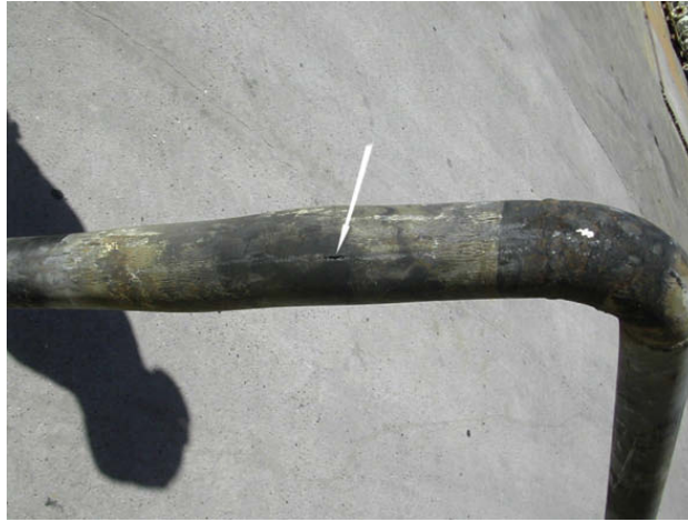
Fig. 1. Failed section of the pipe.
