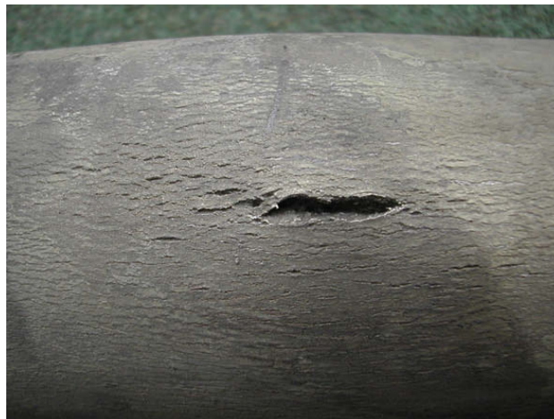
Fig. 2. Failed section of the pipe after cleaning.
