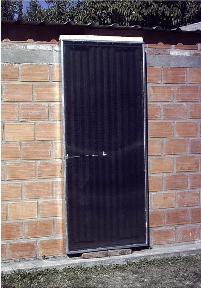
Fig. 3. Solar air collector installed for testing.
