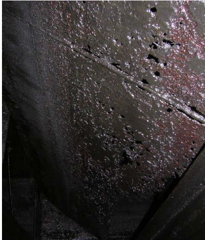
Fig. 5. Photograph showing filter with attack (pitting)
