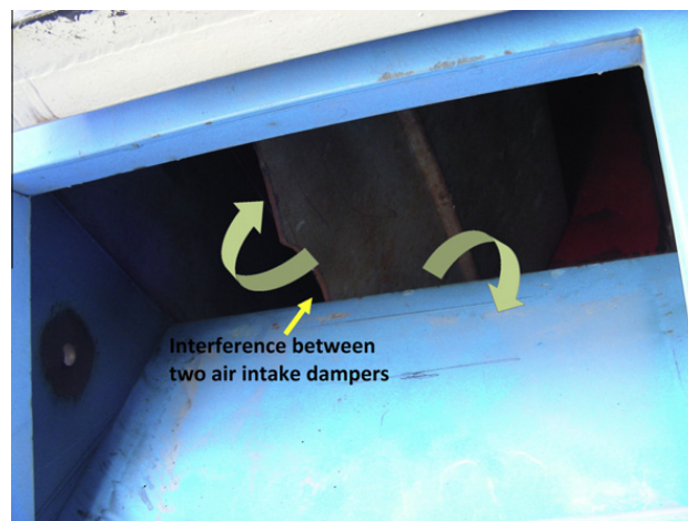
Fig. 7. Intake dampers after cuts done by maintenance staff both gates could get stuck both opened and closed.
