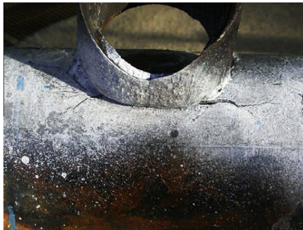
Fig. 3. Origin of failure Nipple placed as mechanical protection for thermocouples.
