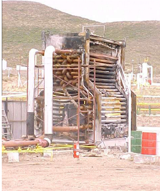
Fig. 2. Fire in a propane, butane and gasoline recuperation and dehydration heater.
