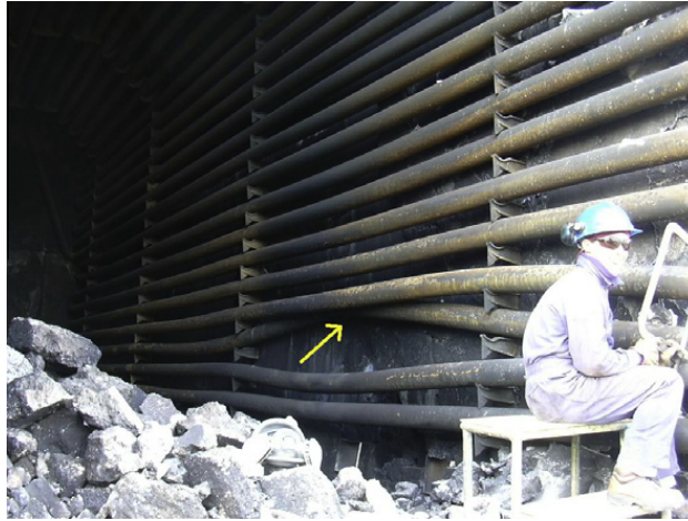
Fig. 4. Leak in a tube near the bottom of a JP1 heater that resulted in a fire.
