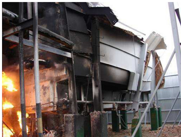
Fig. 9. Location of the fire subsequent to the initial explosion
