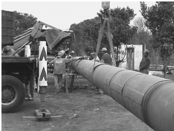
Fig. 1. A tract of pipe with multiple sleeve repairs being prepared for hydrostatic burst testing.
