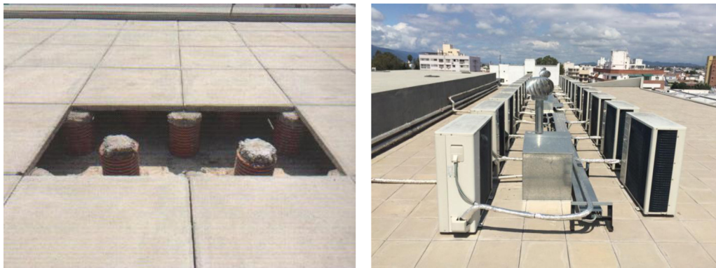
Fig. 5. Rooftop technology (left) and individual air conditioner units (right).
