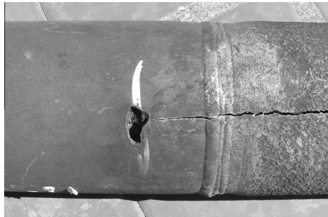
Fig. 2. Open longitudinal crack, arrester to stop crack propagation.
