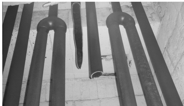
Fig. 1. Failed tubes within the furnace after emergency stop.
