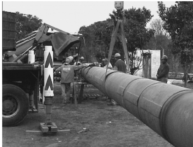
Fig. 9. A tract of pipe with multiple sleeve repairs being prepared for hydrostatic burst testing [28].
