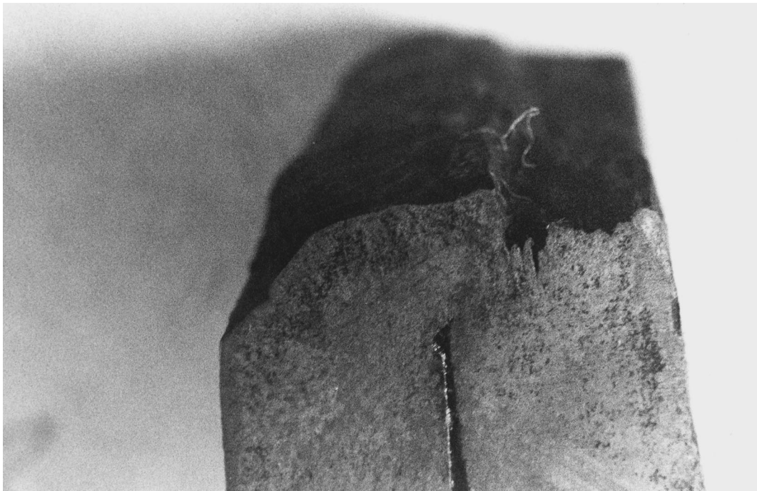
Fig. 7. Cross section of fractured weld in Failure 2. Note the stepped nature of the fracture, with perpendicular secondary cracks into sleeve base material.
