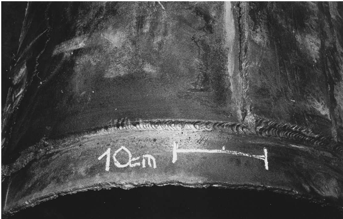
Fig. 4. Circumferential weld of fractured full encirclement repair. Note single pass fillet welds, and longitudinal crack ending close to the circumferential weld.
