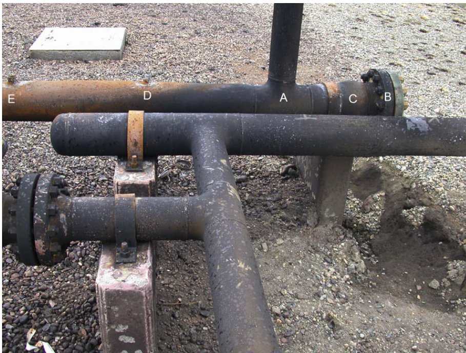
Fig. 2. 8 in. lower suction pipe. (A) End Tee for vertical pipe, (B) end flange, (C) strong deformation, (D) cap to thermometer, (E) cap to manometer.
