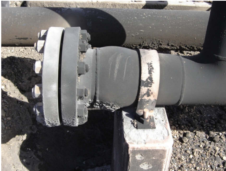
Fig. 3. Deformed tract (detail C in Fig. 2), as seen immediately after the fire.
