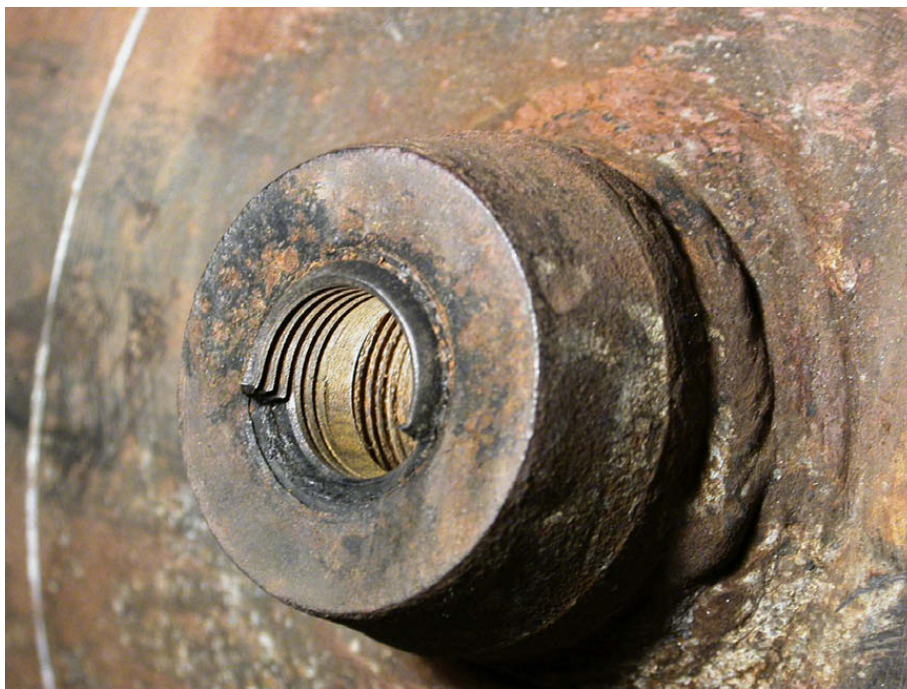
Fig. 7. Fracture at thread in weldolet of manometer (E, Fig. 2).
