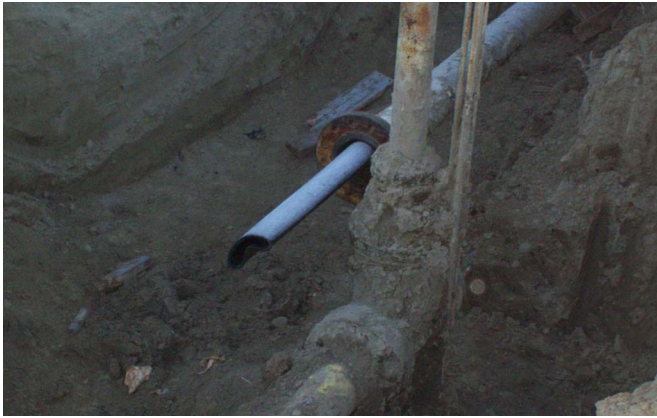
Fig. 1. In-service liner buckling collapse.
