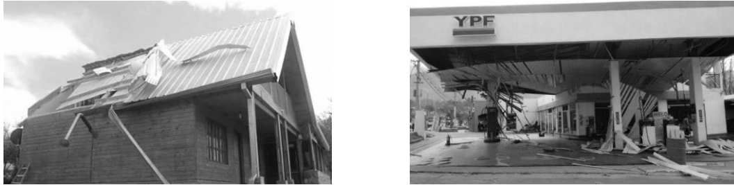
Fig. 4 Roofs damaged by the Zonda wind event on August 5 th , 2015
