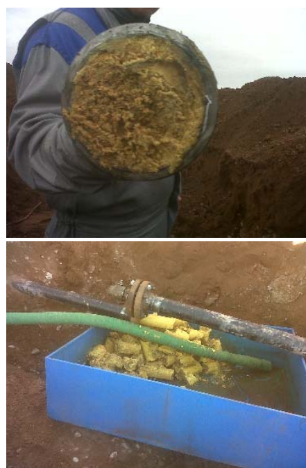
Fig. 1 Pipeline obstruction at YPF's "Loma La Lata Norte" location
