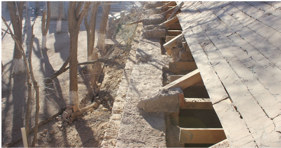
Fig. 7 Details of the reinforced concrete beam incorporated into the adobe walls (Source: the authors)
