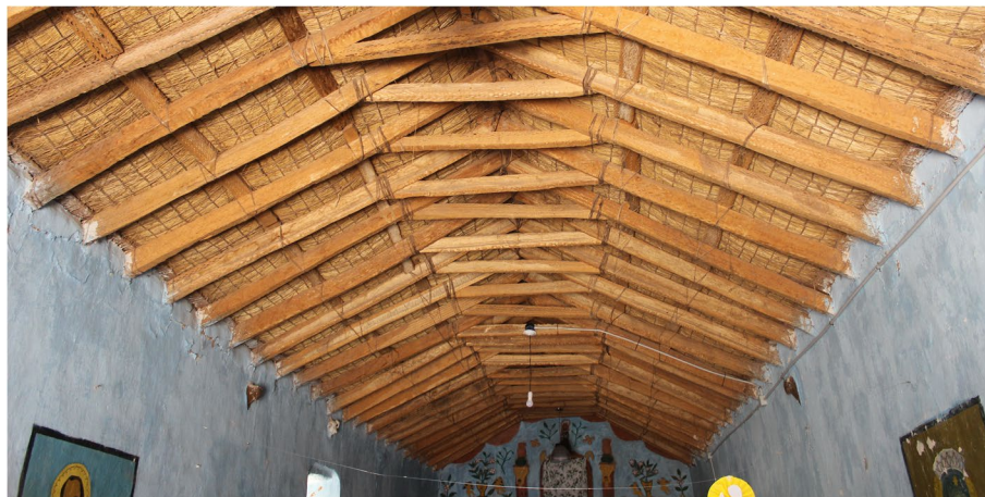
Fig. 5 Details of the cardon wood and thatch roof seen inside the nave (Source: the authors)
