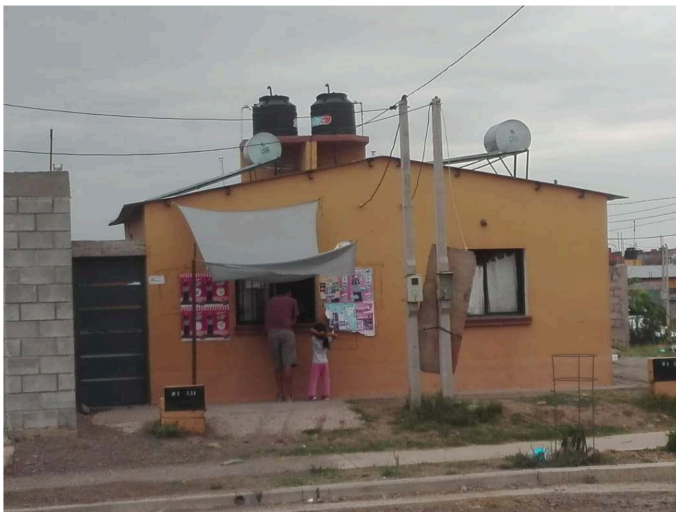
Photo 2. Solar water heaters in social neighborhoods of San Salvador de Jujuy
