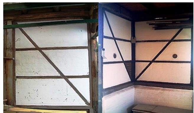
Fig. 16. Actual state of E. W's wattle and daub North walls
