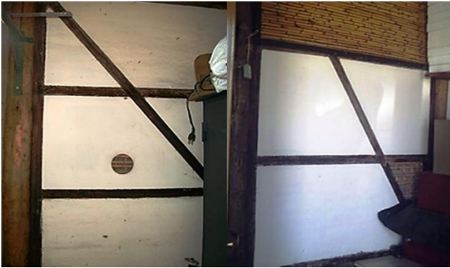
Fig. 17. Actual state of E. W's wattle and daub South walls
