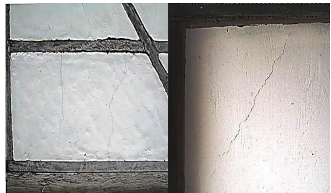
Fig. 15. Micro cracks on wattle and daub walls.
