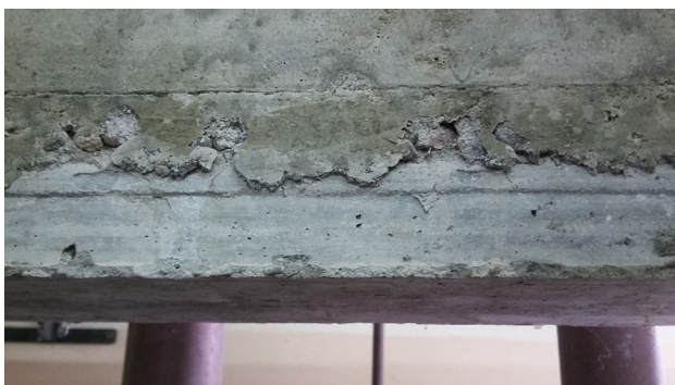
Fig. 12 Zone of the crack in Beam 01 after unloading. The crack is closed and not visible
