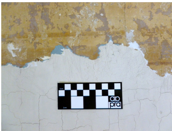
Figure 1 Wall with deteriorated sector in one of the corridors of our research institute
